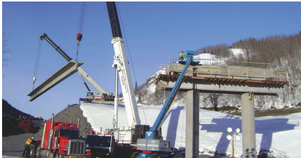
Picking a bulb-tee girder for winter construction of the Hicks Creek Bridge.
